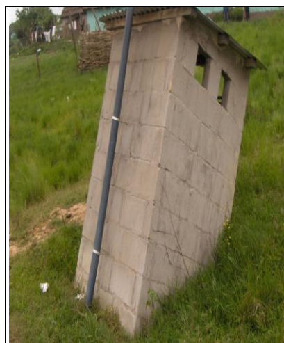
VIP Sanitation Collapsing as no lining provision was made
