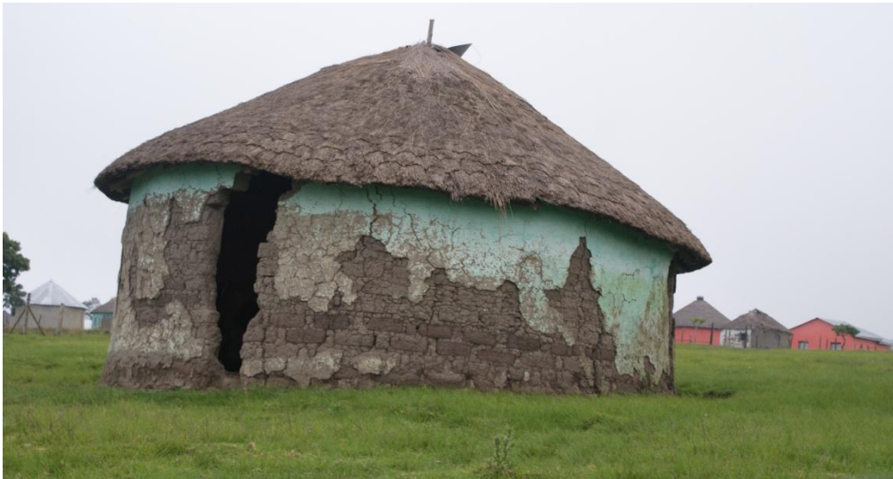
Picture 1: Dilapidated traditional rural dwelling
